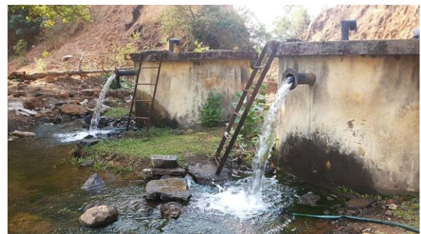
Photo: Wastage of water
